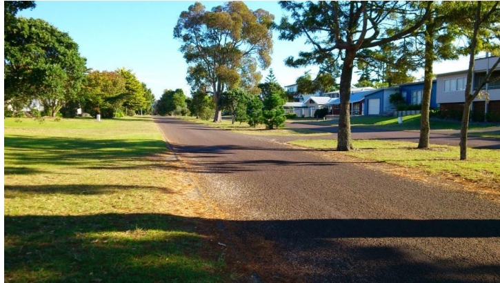
Figure 33: Vista Paku - missing footpath south of Royal Billy Point
