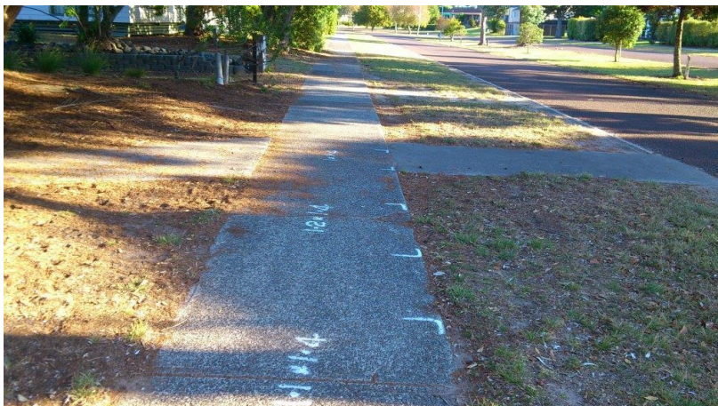
Figure 40: Footpath repair marks on Vista Paku
