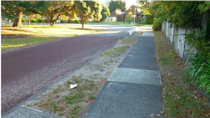
Figure 39: Lifting footpath on Pauanui Boulevard – east of Vista Paku/Hikuai Settlement Road
