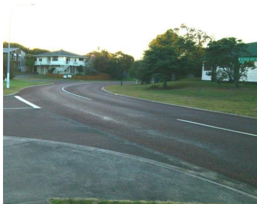
Figure 34: Missing footpath on Pauanui Boulevard
