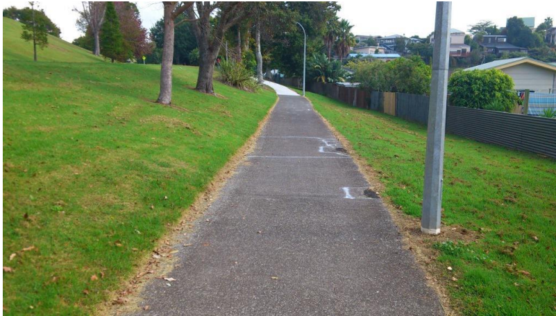
Figure 30: Broken footpath identified for repair
