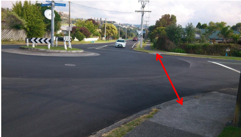
Figure 14: Kerb ramps at Martyn Road force users into the live traffic lane
